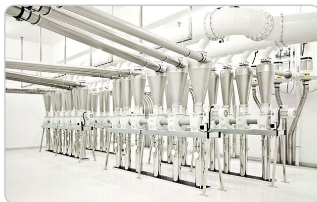
Mill pneumatics and aspirations shall be adjusted via auto-control loops to meet exact pressure and air flow needs.
