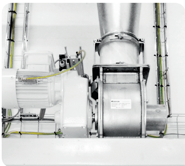
Pneumatic mill stock conveying system: airlock table with cyclone and discharge airlock MPST.
